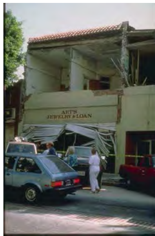
Photo: Collapse of wall of second story of Art's Jewelry and Loan establishment on Greenleaf Avenue in "Uptown" Whittier (Source: NOAA)
