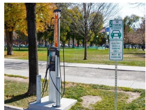
Electric Vehicle Charging Station illustrative
