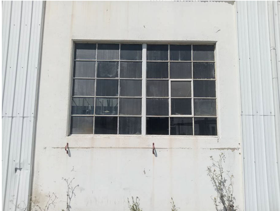
Photograph 7: View of window detail on the original 1950s warehouse. Note the aluminum panel patchwork on the exterior walls of the warehouse.
