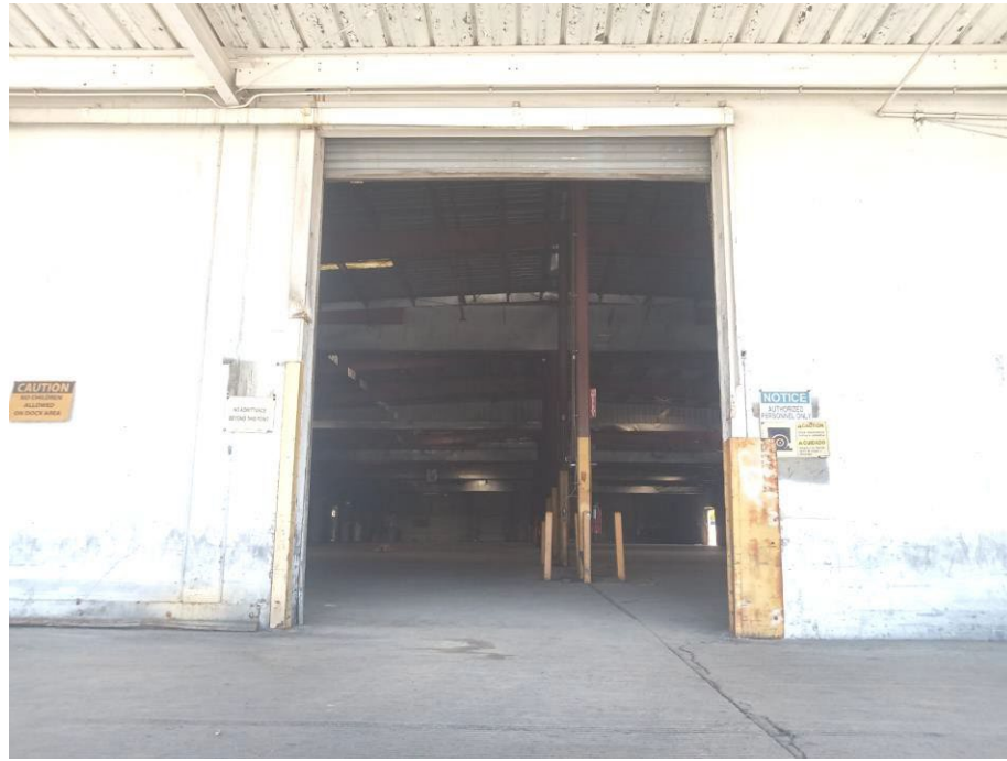
Photograph 13: View looking in the interior of the warehouse through the large bay opening at the trusswork supporting the roof.
