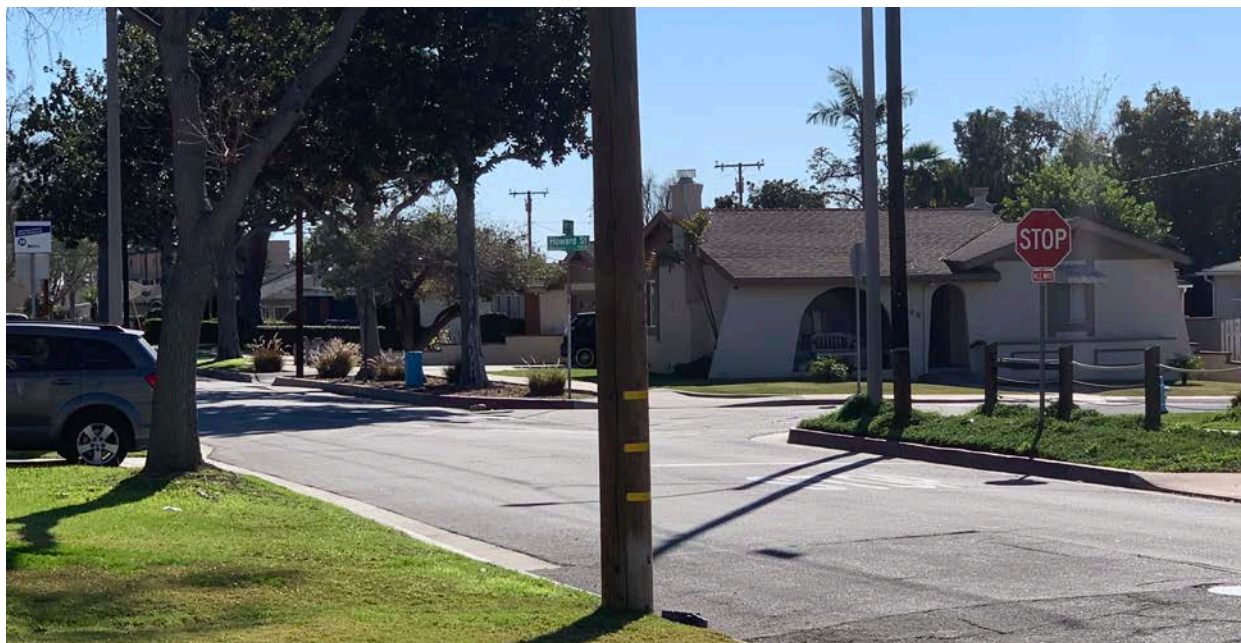
Exhibit 1 - The Corner of Palm Ave & Howard (Greenwood Trail) Notice the paint has worn off 80%
