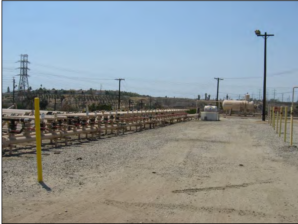
Oil Well Test Station Example
