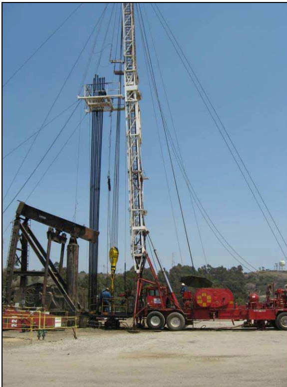
Maintenance Workover Rig
