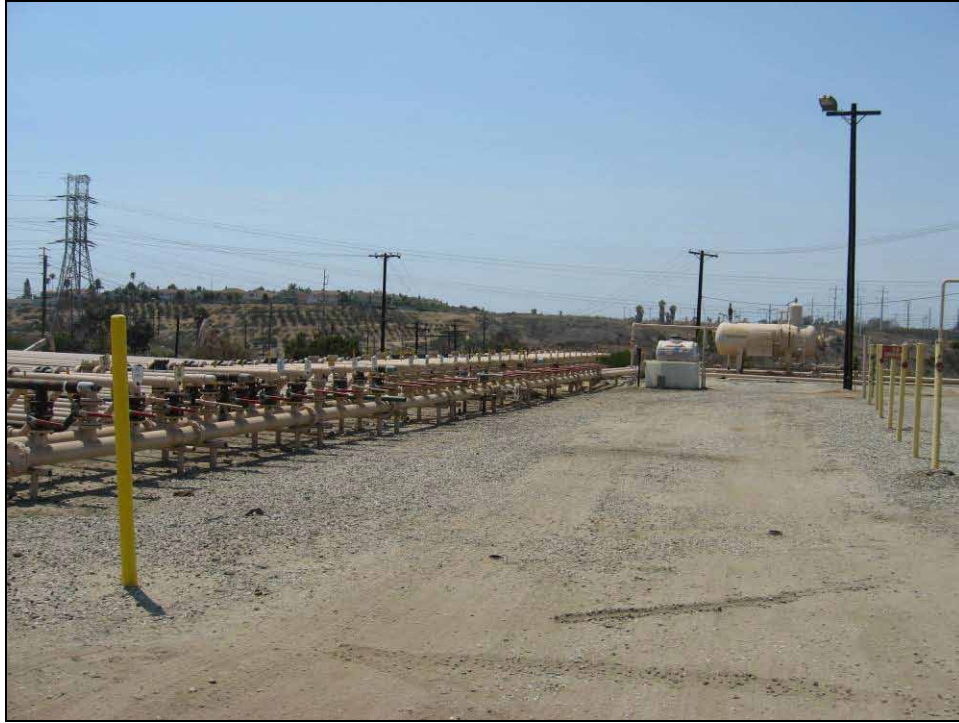
Oil Well Test Station Example
