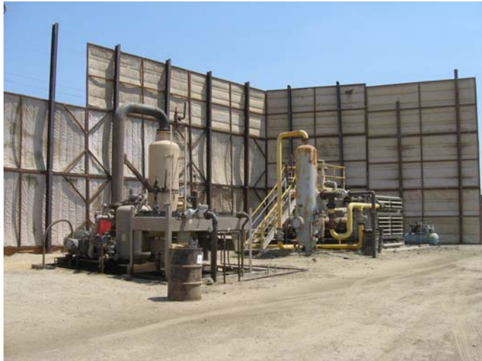
Sound Barrier Wall Around Equipment
